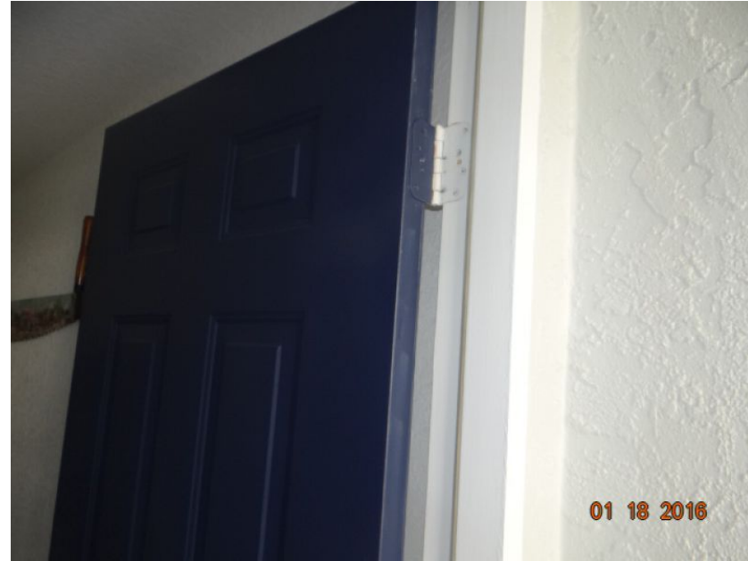
Unprotected Solid Entry Door
