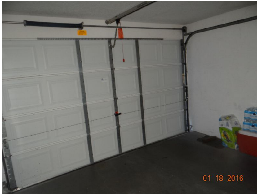
Unprotected Solid Garage Door
