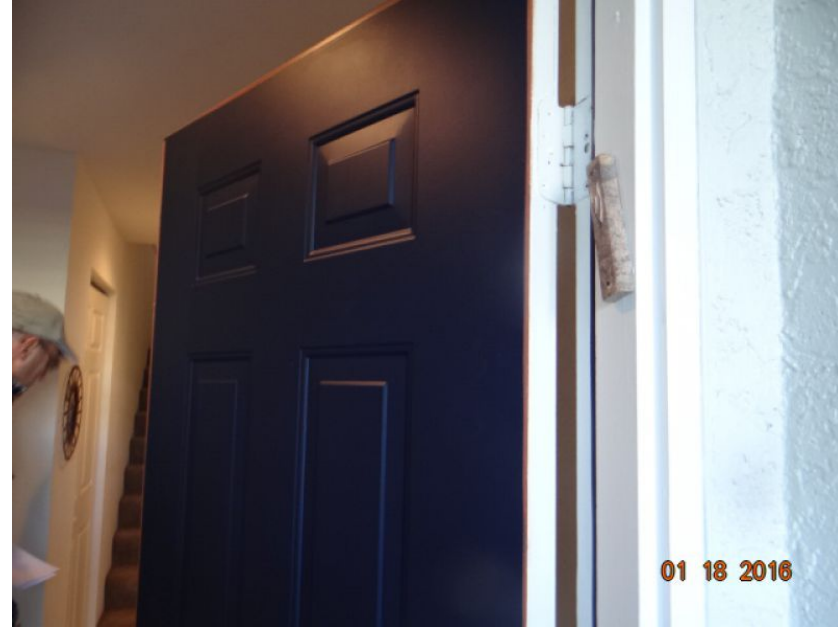
Unprotected Solid Entry Door
