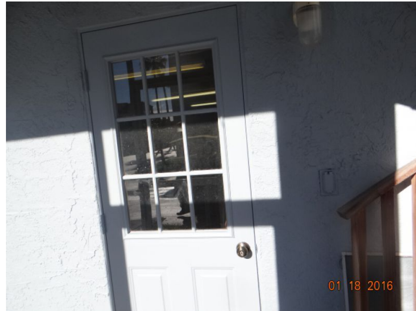
Unprotected Glazed Entry Door
