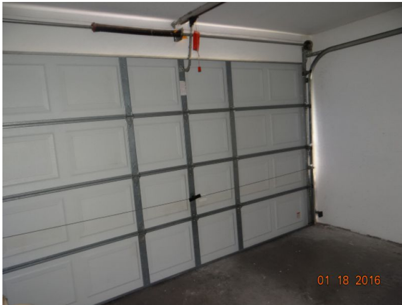
Unprotected Solid Garage Door
