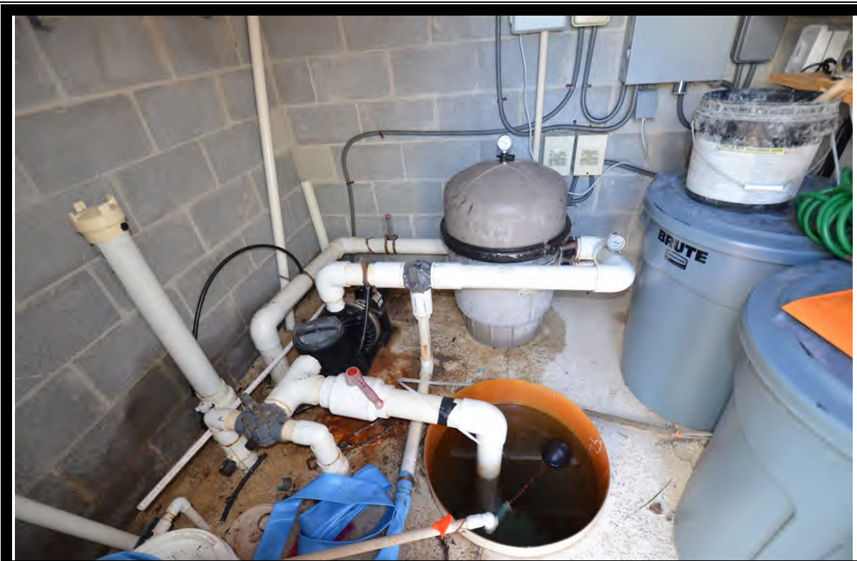
VIEW OF TYPICAL POOL EQUIPMENT
