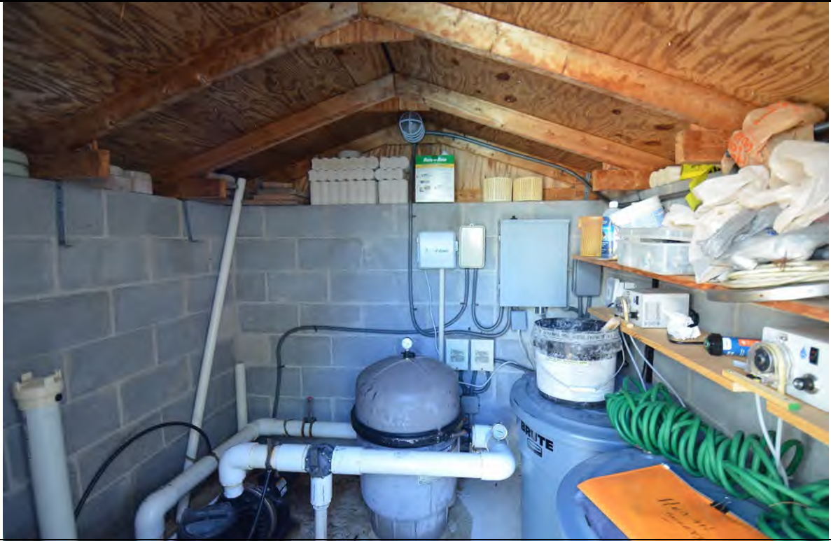
VIEW OF PUMP HOUSE AND TYPICAL POOL EQUIPMENT
